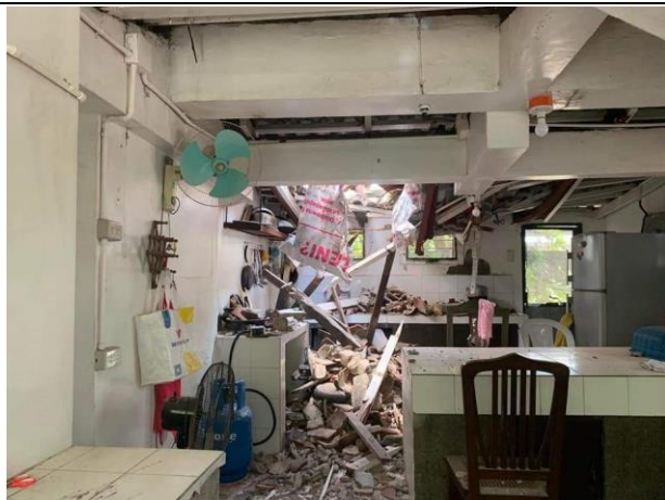
Partially destroyed house in Vigan City, Ilocos Sur
