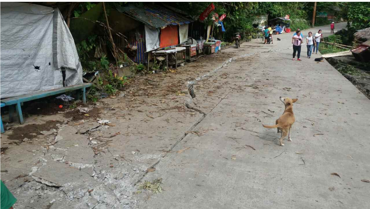
Photo 3. Big cracks are seen on a barangay road in Danao, Ormoc City (Photo by Reniel Lero)
