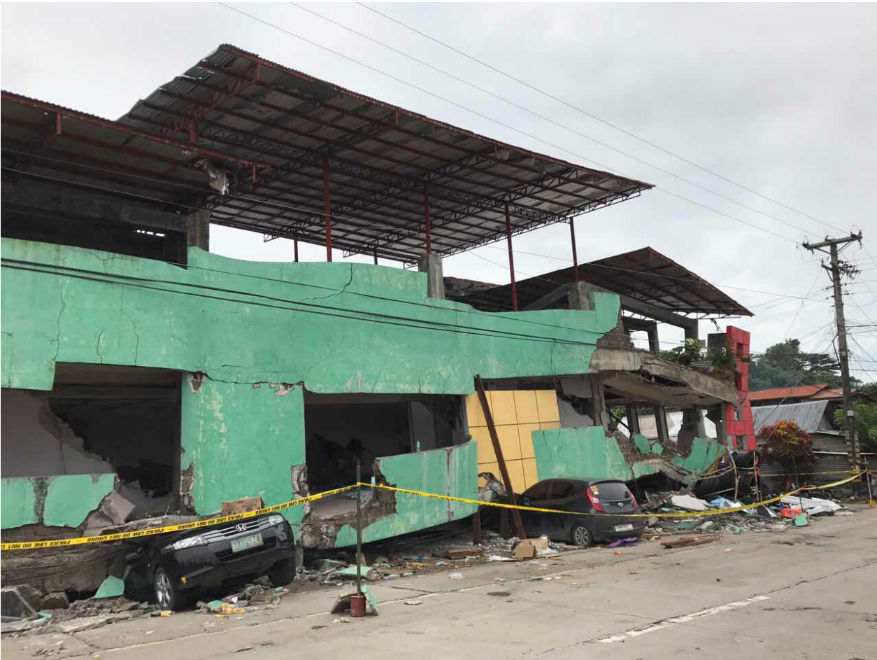
Photo 2. The 3-storey pension house that collapsed in the town of Kananga. (Photo by Margarito Costelo)
