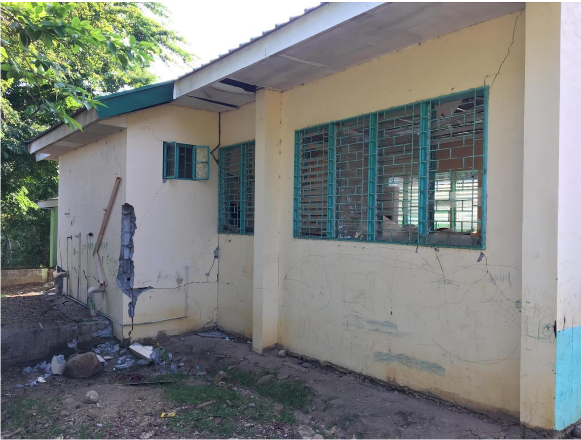
Photo 7. Damaged classrooms at Camias High School (Marvin Natividad).
