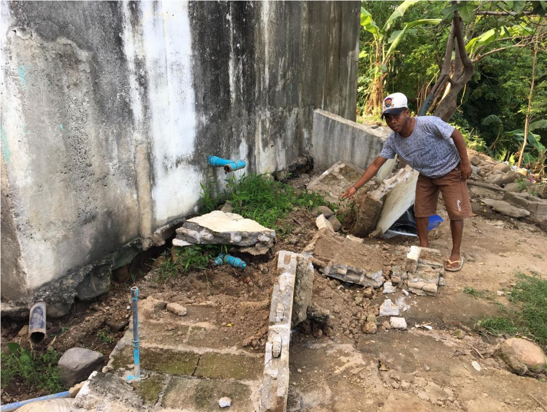
Photo 8. Damage noted at water reservoir in Porac (Marvin Natividad).
