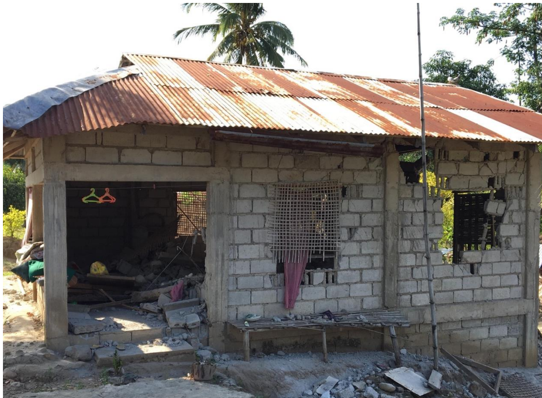
Photo 9. Partially damaged house (Marvin Natividad).
