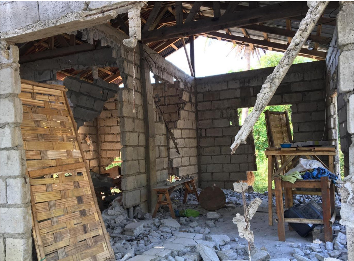
Photo 11. Totally damaged house (Marvin Natividad).
