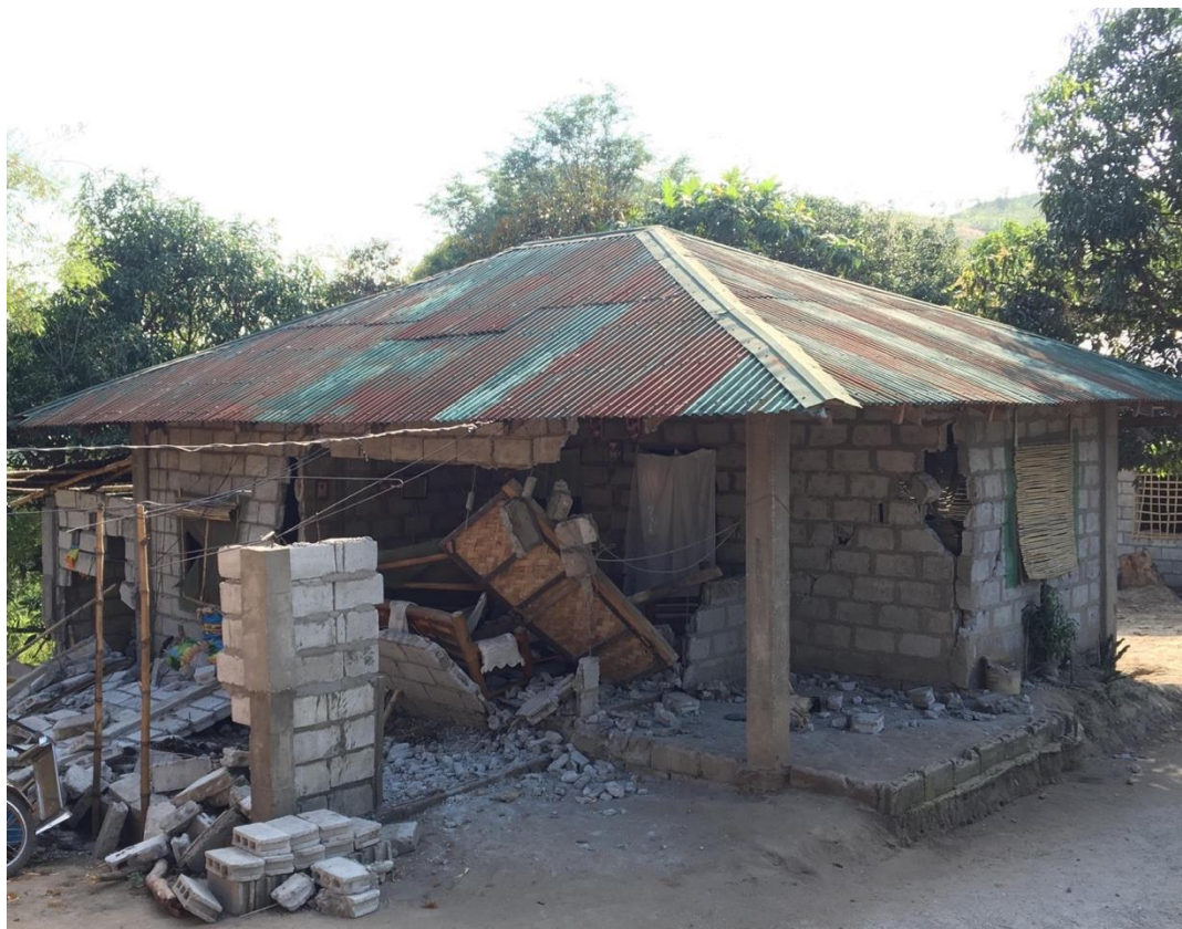
Photo 10. Still standing but with severely weakened pillars (Marvin Natividad).
