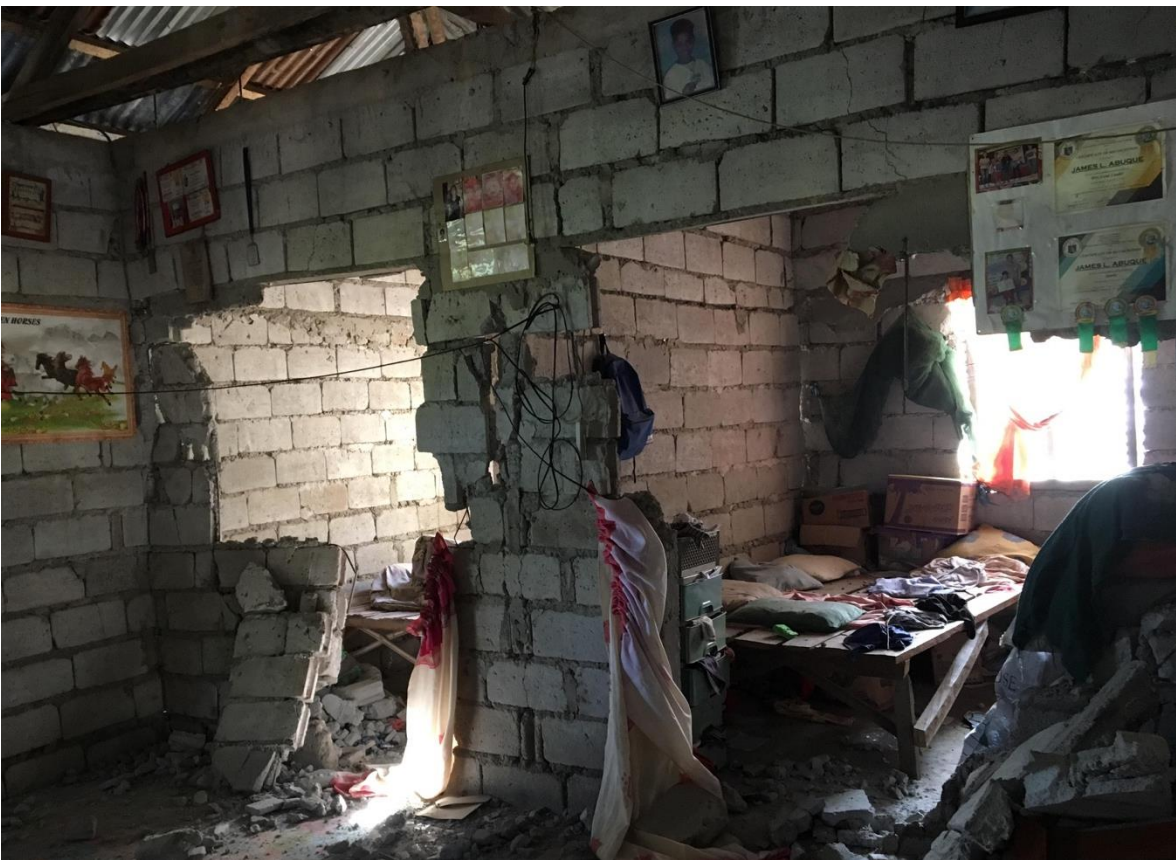
Photo 12. Damaged house vacated by residents (Marvin Natividad).
