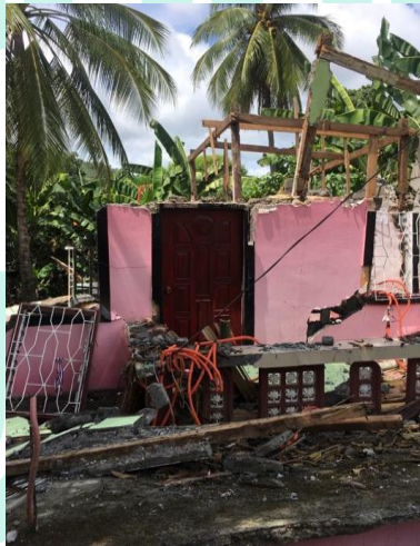
Damaged house in Malawanit.
